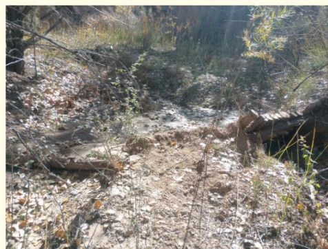
A log rack (or trash rack) from local juniper posts (on right side in image) that has captured sediment and sends flows off to the "right-bank" of the channel (on left side in image) where logs create a sill that holds the grade.
